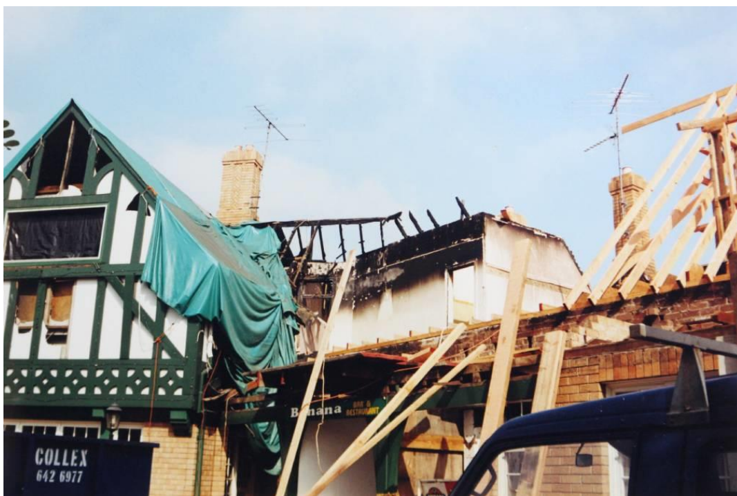
Figure 14 - Extensive fire damage in 1991 prior to reconstruction
